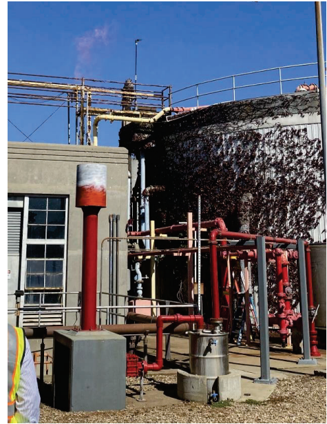
Figure 1 Existing WPCP Gas Flare
