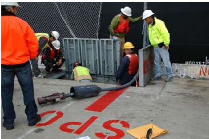
Shore power outlet
