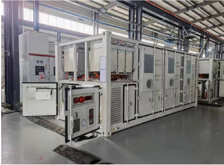
Figure 1 Sample Battery Energy Storage System (BESS)
