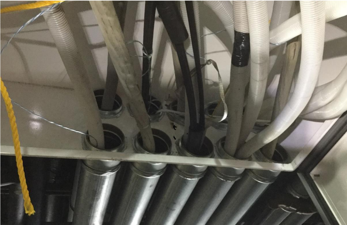
Picture 2: Inside of the second pull box after the pull room. (Marked "2" on the attached drawing)
