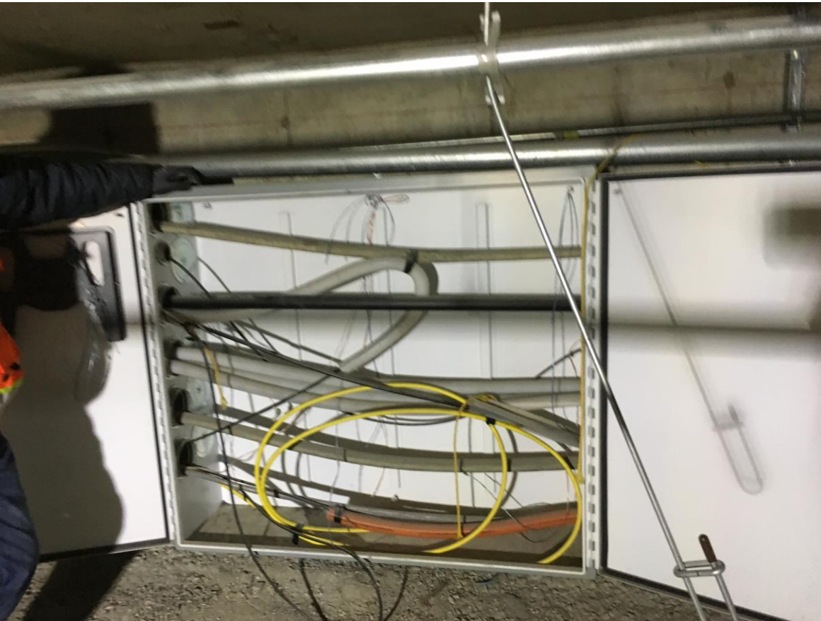
Picture 3: Unvisited Pull box in the Basement of M102 building.
