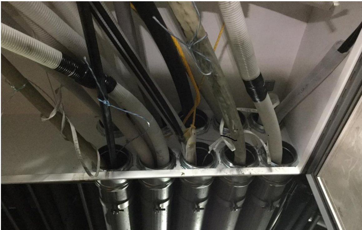
Picture 1: Inside of the first pull box after the pull room. (Marked "1" on the attached drawing)
