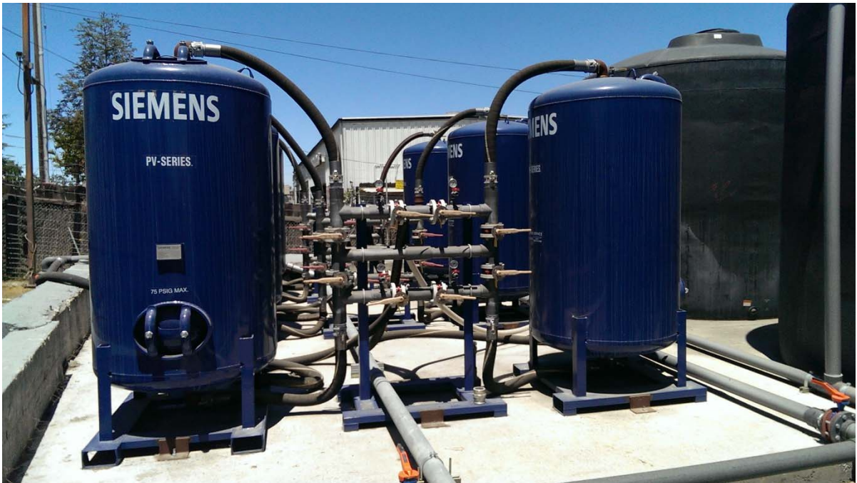
Filtration and Carbon Polish (Backwash Tank)
