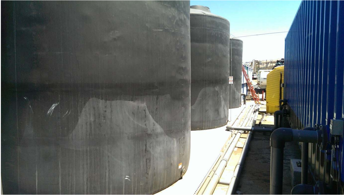
Storage and Preliminary Clarification (Pre-Treatment Tank)
