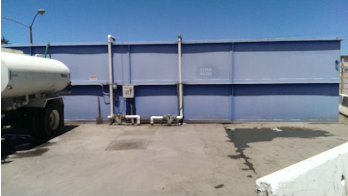
Clarification (Clarifier Tank)
