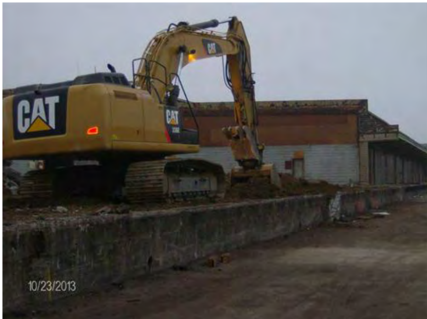
BBGB excavating existing raised slab where building has been deconstructed and removed
